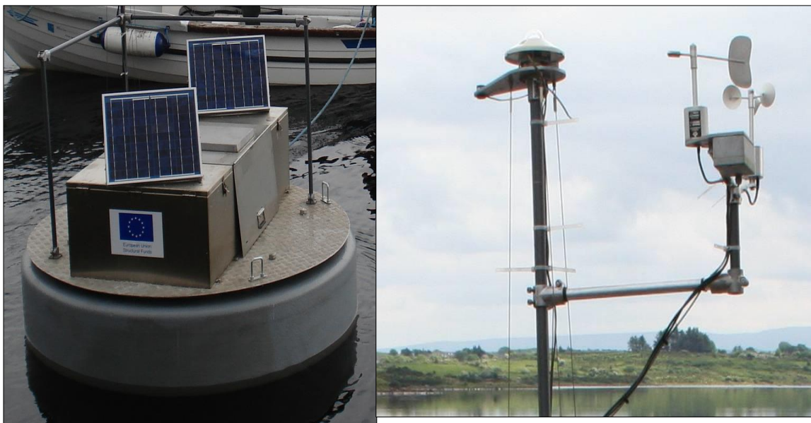
Figure 2-10: The Automatic Water Quality Monitoring Station (AWQMS) on L. Furnace (left) and the meteorological instruments attached (right).
